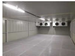
Modular Cold Storage Room
