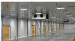
Commercial Cold Storage Room
