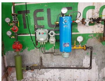
Commercial Gas Pipeline Fitting
