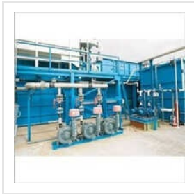
Industrial Sewage Treatment Plant
