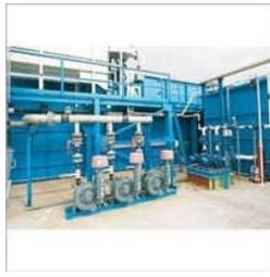
Industrial Sewage Treatment Plant
