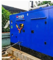
62 KVA Tata Electric Power Generator
