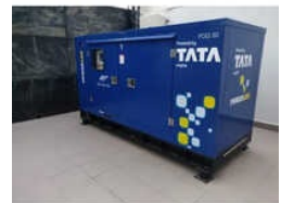
30 KVA Tata Silent Diesel Generator
