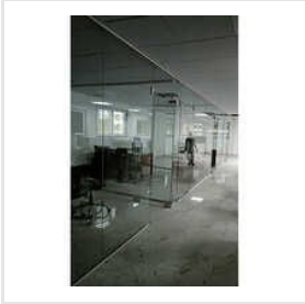
Office Glass Partition
