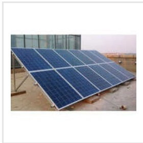
Three Phase On Grid Rooftop Solar Power
