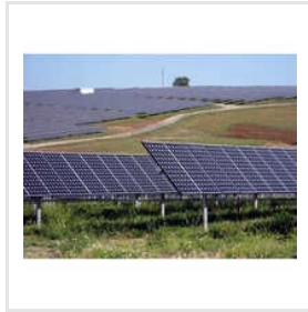
15kW Roof Top Solar Power Plant
