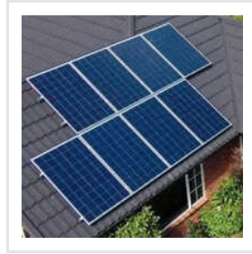
Off Grid Solar Power Plant
