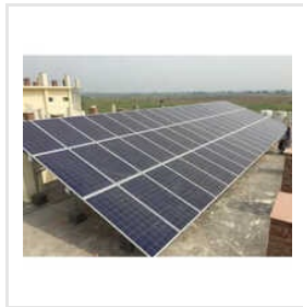
40kW Solar Power Plant
