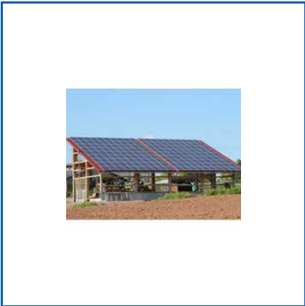
ROOFTOP SOLAR POWER PLANT
