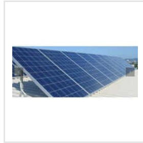
20kW Solar Power Plant
