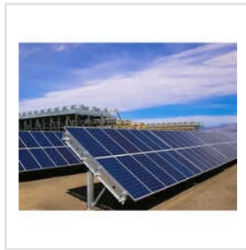
Grid Tied PV Solar Power Plant
