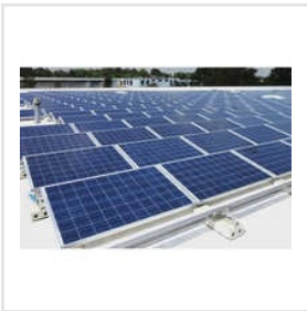
Single Phase Off Grid Rooftop Solar Power
