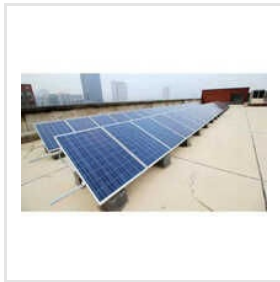
Single Phase On Grid Rooftop Solar Power
