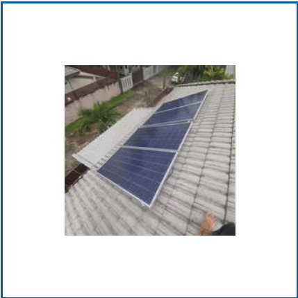
5KW INDUSTRIAL SOLAR POWER PLANT
