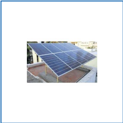
THREE PHASE SOLAR POWER PLANT
