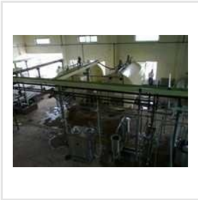
Milk Processing Plant
