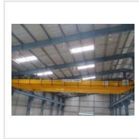
Overhead EOT Double Girder Cranes
