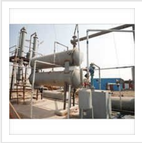
Waste Tyre Recycling Unit (Pyrolysis)
