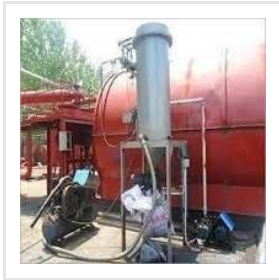
Waste Tyre Recycling To Oil Plant
