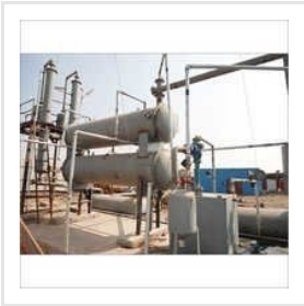
Waste Tyre Recycling Unit (Pyrolysis)
