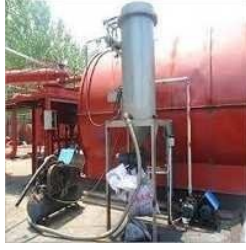
Waste Tyre Recycling To Oil Plant
