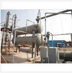
Waste Tyre Recycling Unit (Pyrolysis)
