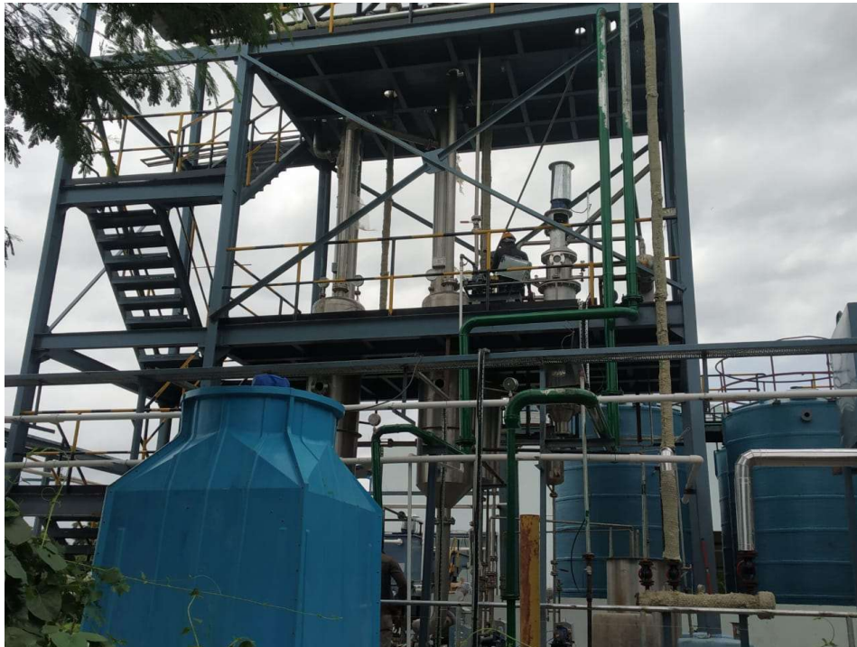
10KPLD plant- Double Effect Evaporator followed by Agitated Thin Film Dryer
