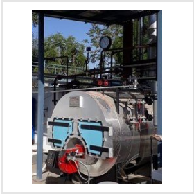
Oil Fired Steam Boiler
