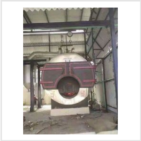
Wood Fired Boiler
