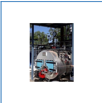
OIL FIRED STEAM BOILER
