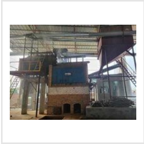
Husk Fired Boiler
