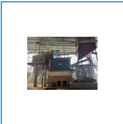
HUSK FIRED BOILER
