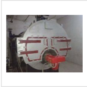
Oil Fired Boiler
