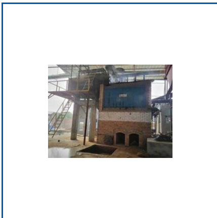
RICE HUSK FIRED STEAM BOILER
