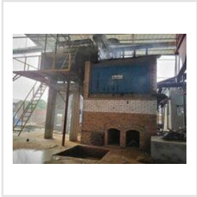
RICE HUSK FIRED STEAM BOILER
