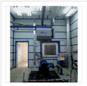
Engine Test Cell Acoustic Lining
