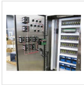
VFD Based Control Panel
