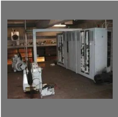
Machine Room Passenger Elevator
