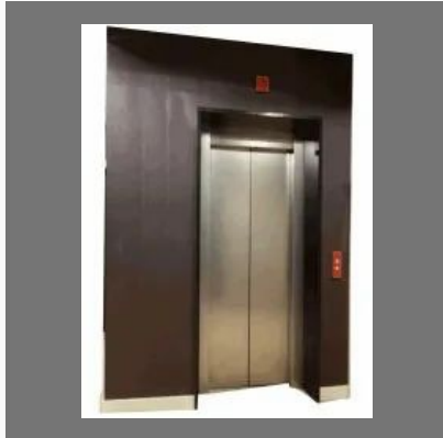
6 Persons Passenger Elevators
