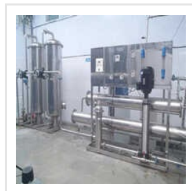
2000 LPH Mineral Water Plant
