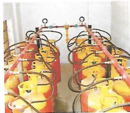
Gas Pipe Line KD-EH-09
