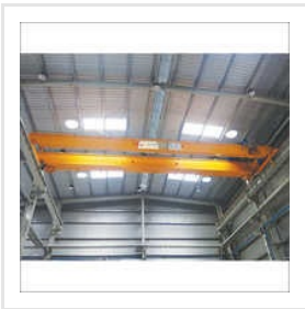
Double Girder Eot Crane
