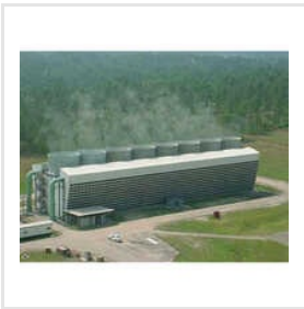
Industrial Cooling Tower Chemical Plant
