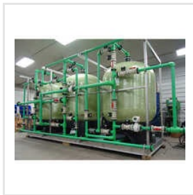
Filtration And Softeners Plant
