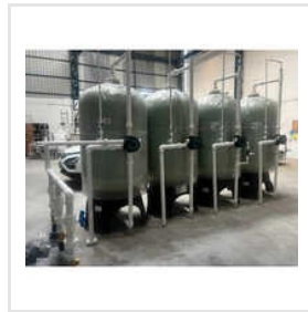
Pre Filtration Plant
