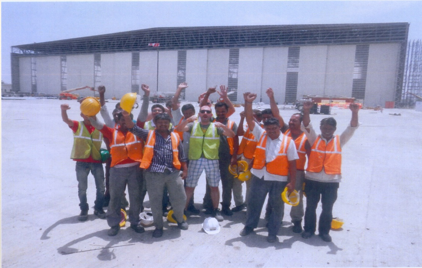
A MIHAN PROJECT AT NAGPUR-ERECTION OF DOUBLE HANGAR DOOR, 200.0M WIDE WITH 8 FLAPS OF 25.0M & 27.0M HEIGHT; 4 FLAPS EACH ROLLS ON EITHER END IN OUT RIGGER, EACH DOOR FLAP IS WEIGHING 58.0 M/T (+)
