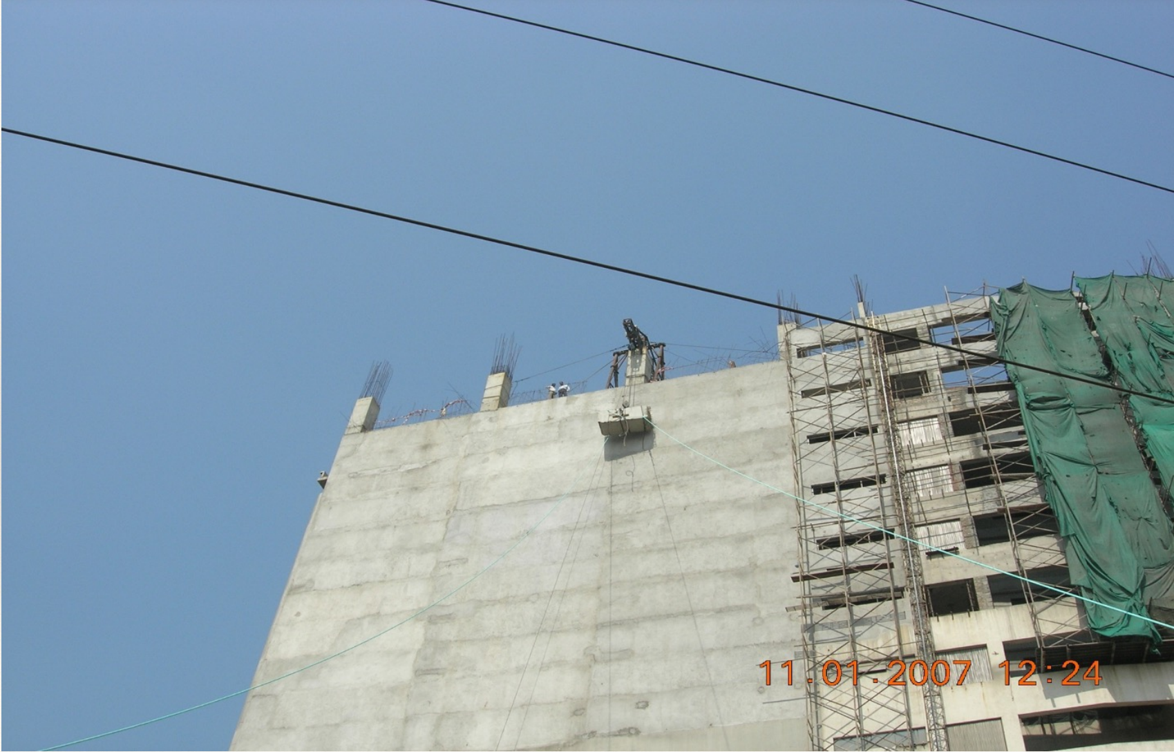
A CUT-OUT RCC COLUMN PIECE IS BEING LOWERED DOWN WITH MECHANICAL DEVICE FROM A HEIGHT OF 58 METERS.
