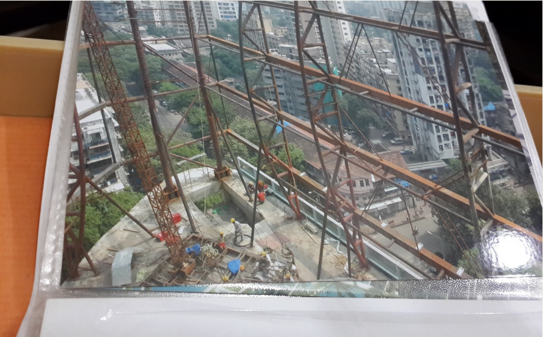
M/S MOTILAL OSWAL, PAREL SITE . FABRICATION OF STEEL SKELETON STRUCTURE FOR SKY LOUNGE ON 8 TH FLOOR HEIGHT 24 METERS . ERECTION WITH THE HELP OF MECHANICAL FABRICATED CRANE ON 8 TH FLOOR SEMI AUTO. CAPACITY 10 MT WITH BOOM HEIGHT 27 METERS.
