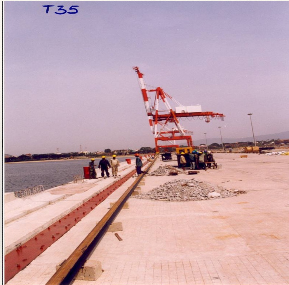
VISAKHAPATNAM - WORKS CARRIED OUT OF FIXING OF SOLE PLATE, CABLE TRENCH AND LAYING & FIXING OF CRANE RAIL.
