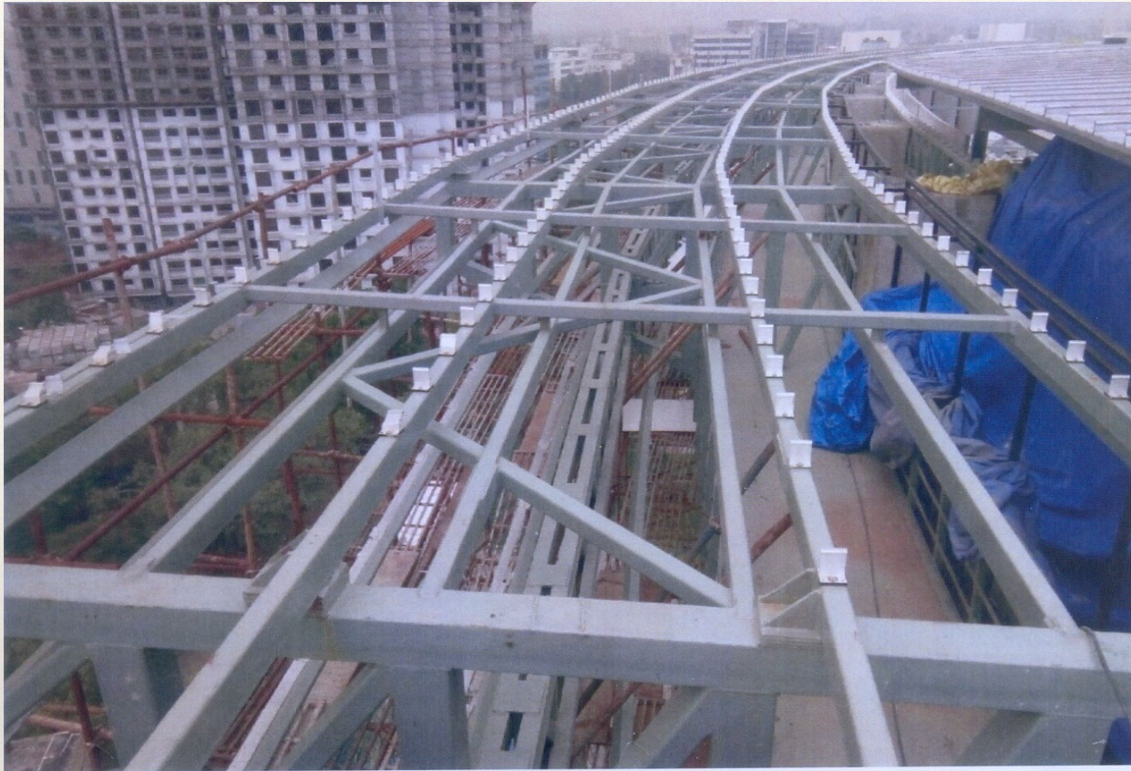
FABRICATION & ERECTION OF ROOF LEVEL CANOPY IN CIRCULAR ARCH WITH PROVISION OF MONORAIL FOR THE SYSTEM OF CLEANING OF GLASSES, CAT-WALK & PROVISION OF RUNNERS FOR ROOF KALZIP SYSTEM AT K.RAHEJA PLATINUM, MAROL, ANDHERI, MUMBAI.
