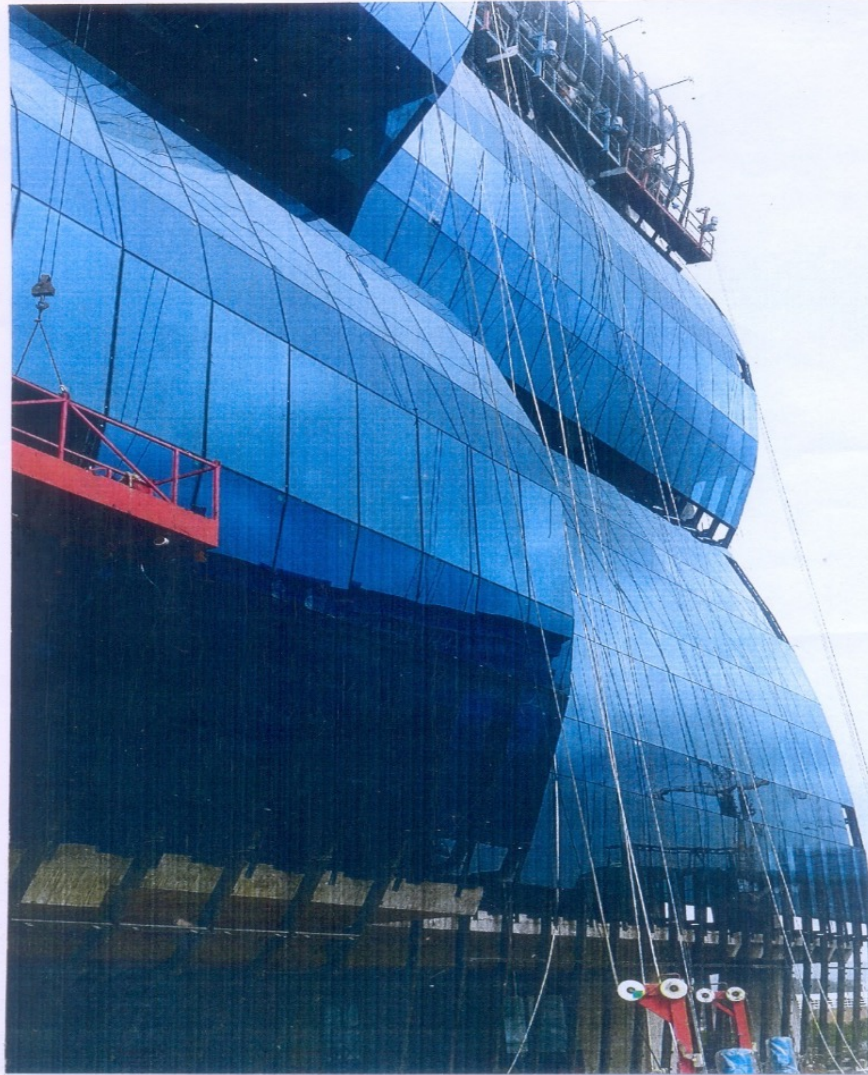
FABRICATION OF SKELETON STEEL STRUCTURE SUPPORTING GLASS FAÇADE & ERECTION AT INS BUILDING CONSTRUCTION BANDRA-KURLA COMPLEX, BANDRA, MUMBAI. IT HAS 6 DIFFERENT CURVES + 1 'S' CURVE AND EITHER SIDE 3 DIFFERENT SIZES OF VASES.
