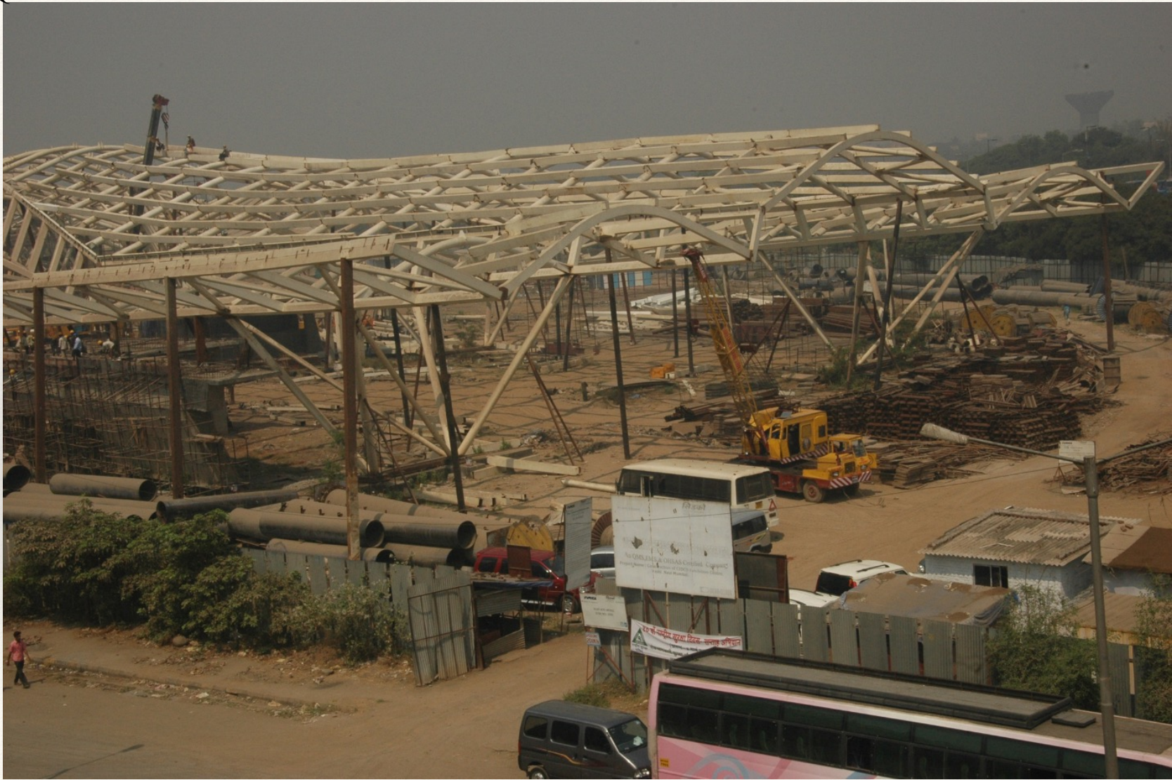
CIDCO EXHIBITION PAVILION, VASHI, MUMBAI . WORK SITE. FABRICATION AND ERECTION OF STEEL SKELETON STRUCTURE. QUANTITY 1200 METRIC TONNES
