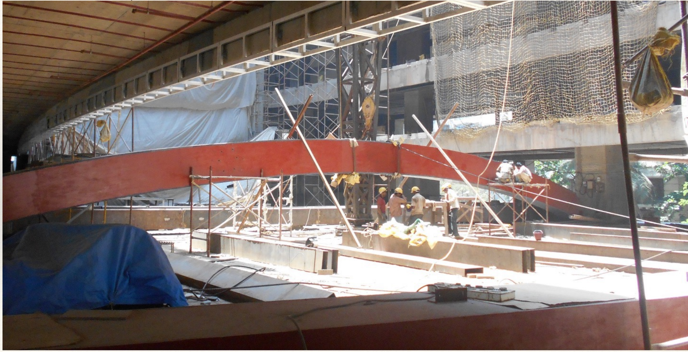
NMIMS WORKS SITE AT VILLE-PARLE, MUMBAI . ERECTION OF ROOF GIRDER WEIGHT 20 TONES, SPANNING MORE THAN OPENING, BEING LIFTED WITH THE HELP OF 50 TONNE CAPACITY DERRICK AND MECHANICAL DEVICE.
