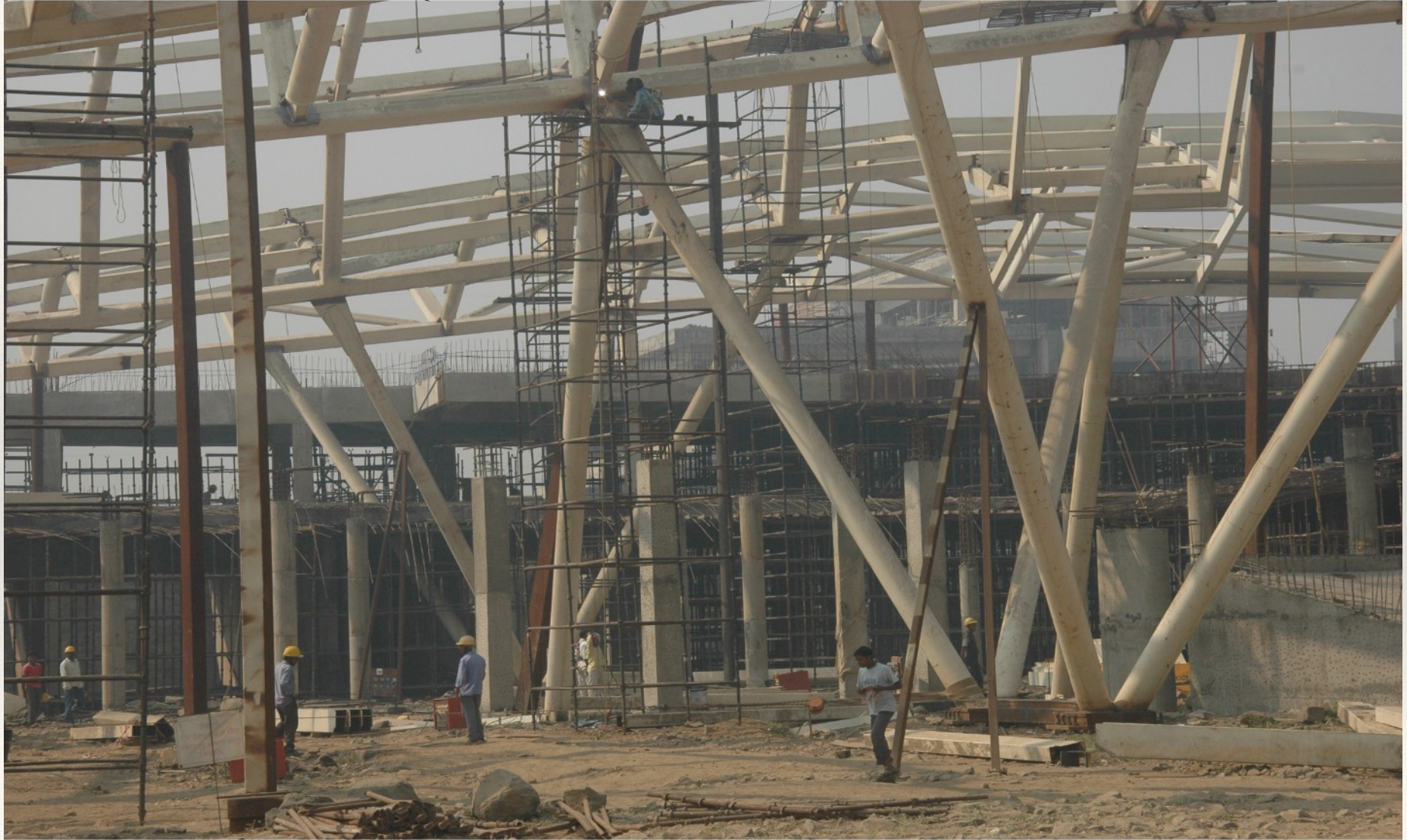
CIDCO EXHIBITION PAVILION, VASHI, MUMBAI . WORK SITE. FABRICATION AND ERECTION OF STEEL SKELETON STRUCTURE. QUANTITY 1200 METRIC TONNES
