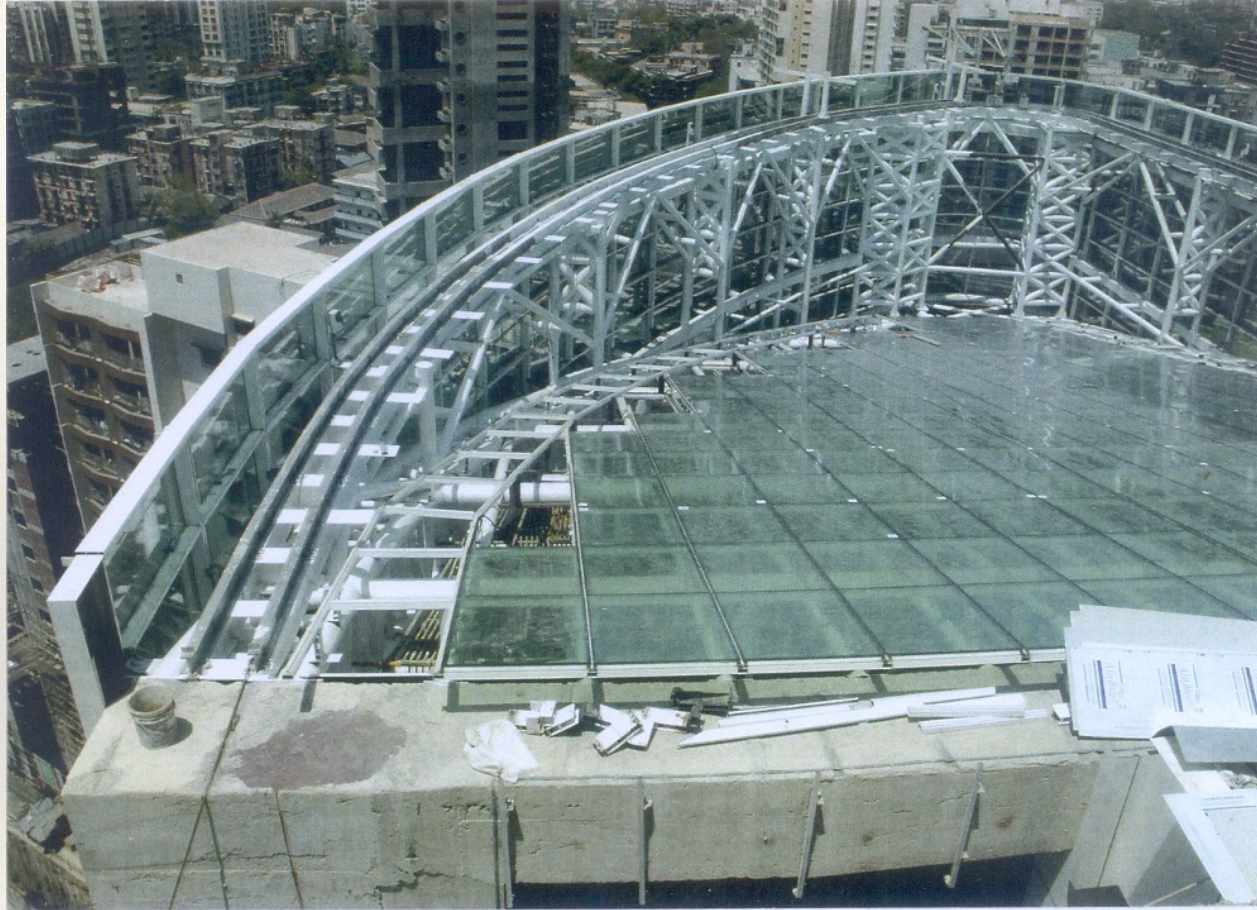
A SKYLIGHT ROOF OVER STRUCTURE INCLUDING GLASS PANELS & TRACK FOR GLASS CLEANING SYSTEM AT MOTILAL OSWAL CONSTRUCTION SITE, PAREL, MUMBAI.
