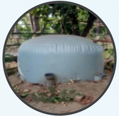
Flexi Balloon Biogas Plant
