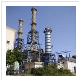
Mild Steel Industrial Chimney
