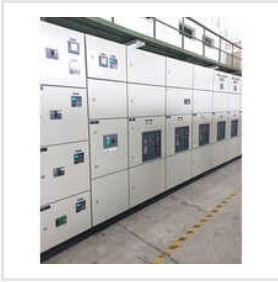
Industrial Synchronization Panel
