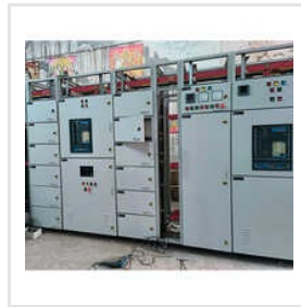
Industrial Load Shedding Panel
