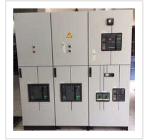
Industrial PCC Panel
