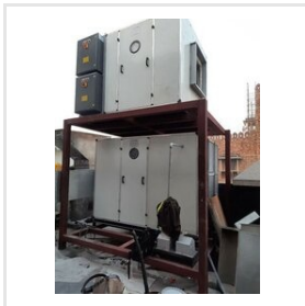
Dry Scrubber Unit
