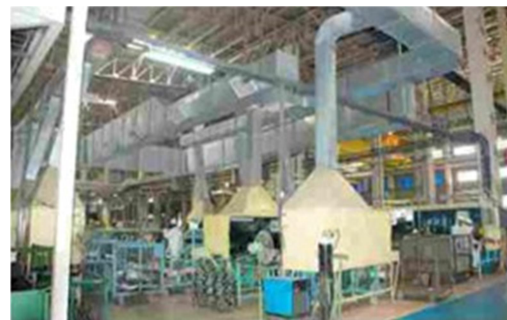
Air cooling of welding shop with fumes Exhaust
