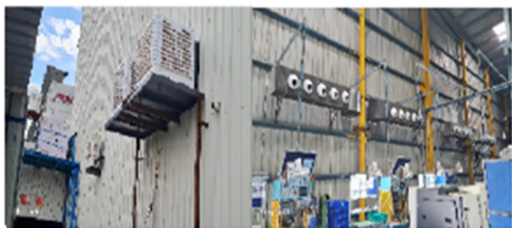
Air Cooler With Ducting
