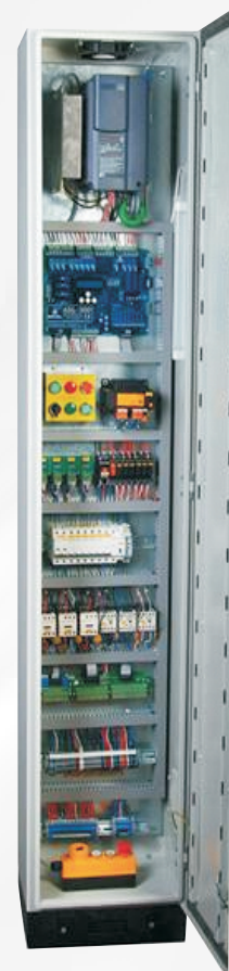
GEARLESS MONARCH POWER CONTROL
