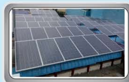
Roof Top Solar Power Plant
