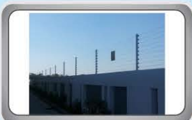
Solar Power Fence
