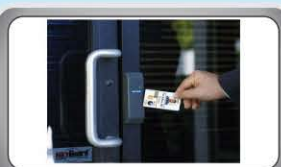
Access Control Interlocking System
