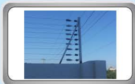
Solar Power Fence
