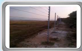
Solar Power Fence
