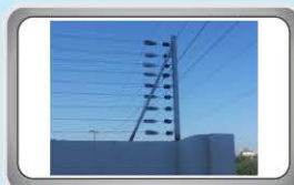
Solar Power Fence
