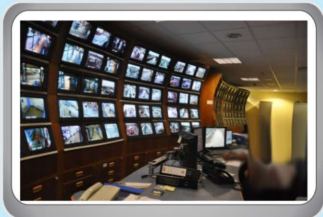
CCTV Control Room
