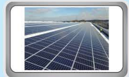
Roof Top Solar Power Plant
