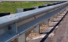
Metal Beam Crash Barrier
