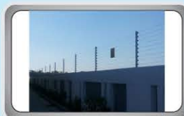
Solar Power Fence
