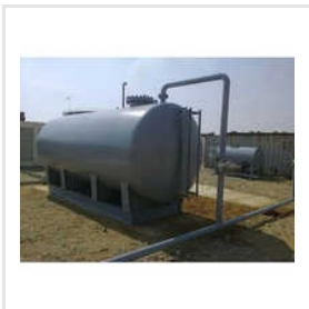
Diesel Underground Storage Tank
