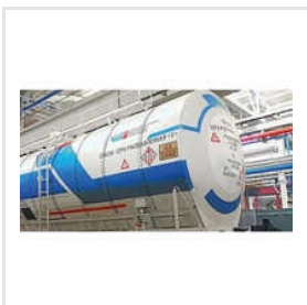
Sulphur Storage Tank
