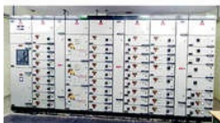
Electrical Control Panel
