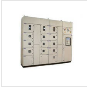
ACB Control Panel
