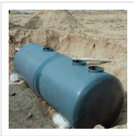
STP Storage Tank
