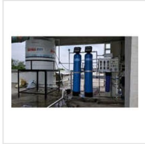
250 LPH FRP RO Plant
