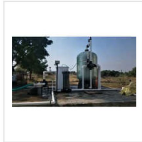
20000 LPH Water Softening Plant
