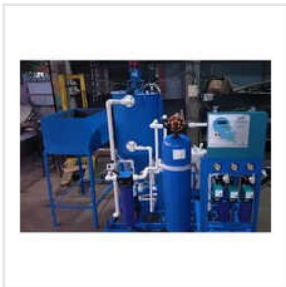
150 LPH Packaged Effluent Treatment
