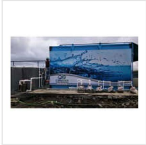
Civil Sewage Treatment Plant
