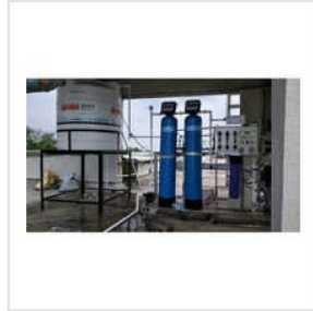
Industrial RO Plant
