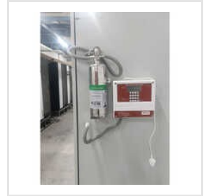
Industrial Fire Suppression System
