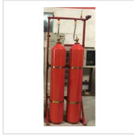
7kg Mild Steel Fire Suppression System
