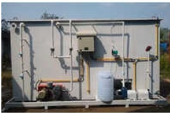
Sewage Water Treatment Plant
