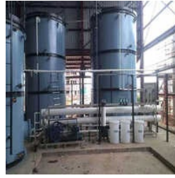
Industrial Zero Liquid Discharge Plant
