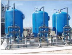
Industrial Water Softener Plant
