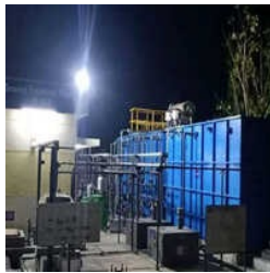
300 KLD Sewage Treatment Plant
