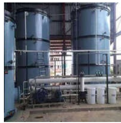
Zero Liquid Discharge System
