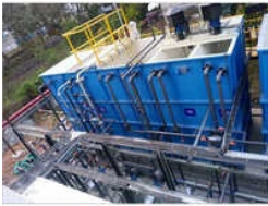
MBBR Sewage Treatment Plant
