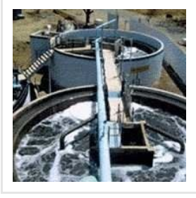
Effluent Wastewater Treatment Plant
