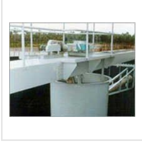
Water Treatment Clarifier
