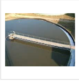
Clean Water Treatment Clarifiers
