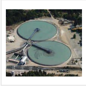
Industrial Waste Treatment Thickener
