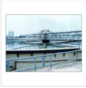
Industrial Reactor Clarifiers
