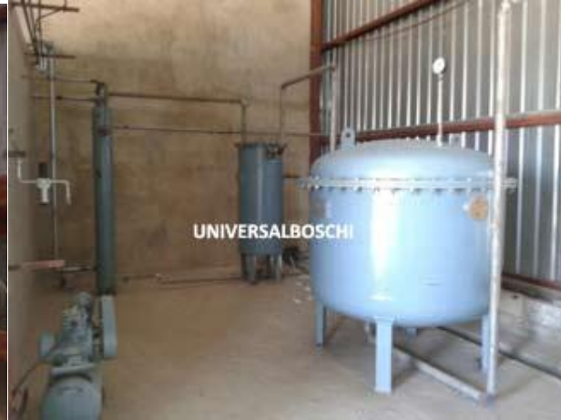
Condenser, L.P Dryer and Purifier
