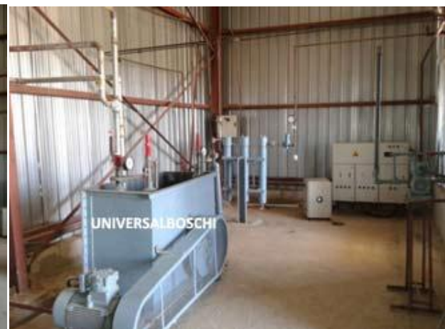
Filling Compressor with control panel
