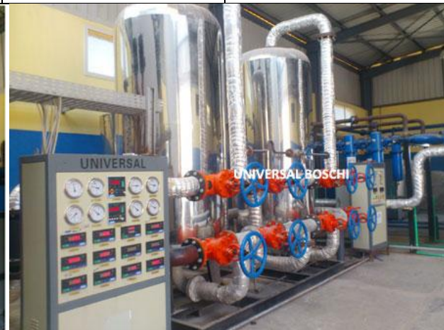
PRE-COOLING PURIFICATION UNIT
