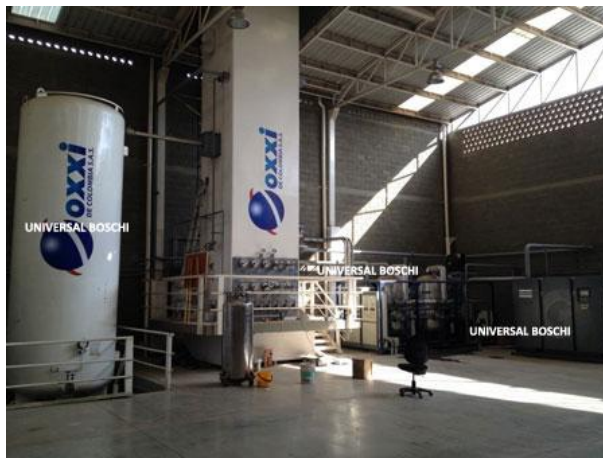
UBTL 50 Ltr/Hr (LIQUID OXYGEN TANK FILLING PLANT)
