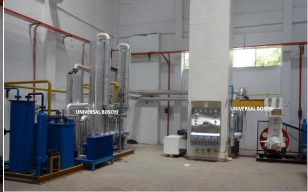
Full View of UBL 80 Liquid Plant
