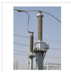
Capacitive Voltage Transformer
