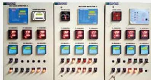
Cold Room Automation Panel
