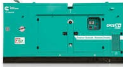
Cummins 750 KVA Diesel Generator
