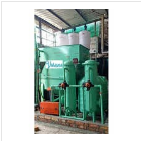
Sludge Treatment Plant
