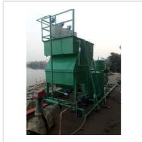
Automatic Sewage Treatment Plant
