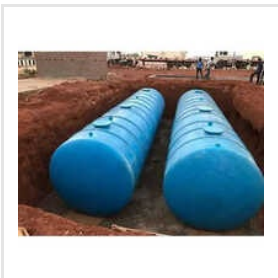
Capsule Sewage Treatment Plant
