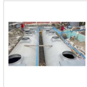
Diaki Sewage Treatment Plant
