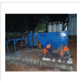
Sewage Treatment Plants For Apartments
