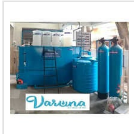
Domestic Sewage Treatment Plant
