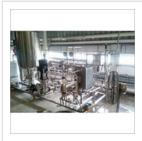
RO Plant With EDI
