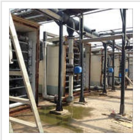
Mobilised Water Treatment Plants
