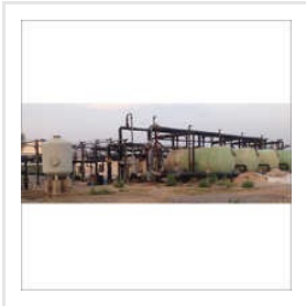
Water Filtration Plants
