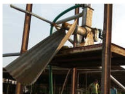
Bio Gas Dewatering Screw Press
