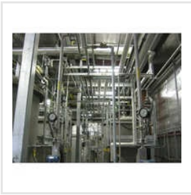
Stainless Steel Process Piping System
