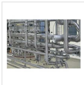
Mild Steel Piping System
