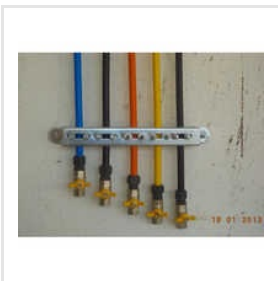
Compressed Air Piping System
