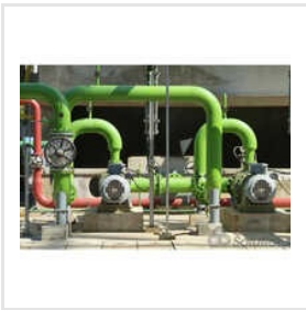
Cooling Water Piping System
