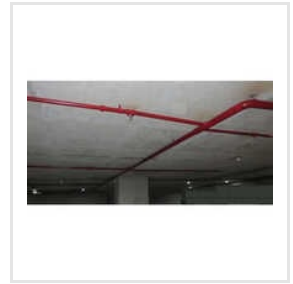
Fire Fighting Piping System
