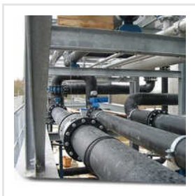
Plumbing Piping System
