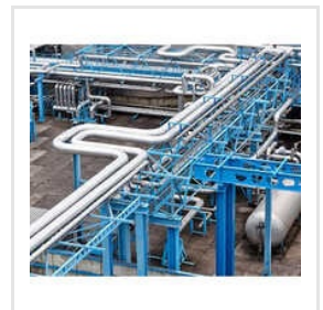
Process Plant Piping System
