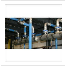
Compressed Air Piping System
