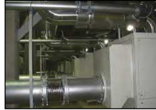
Suji WWTP (NX300), Korea
