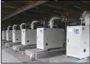
Daejeon WWTP (Nx200), Korea
