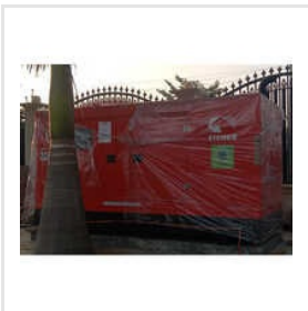
82.5 KVA Diesel Generator
