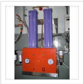
Desiccant Air Dryer
