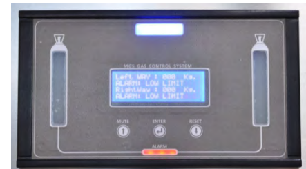
Tube Central Medical Gas Alarm
