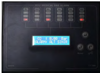
Medical Gas Alarm Panel
