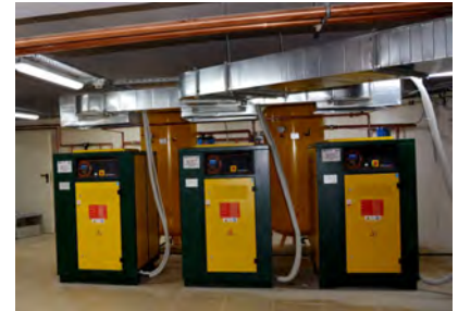
Medical Compressed Air Plant
